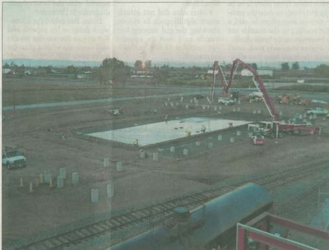
Community Fuels is building a new truck and train loading terminal to handle biodiesel produced at its refinery at the Port of Stockton. Separately, the company announced it will receive a $4.2 million state grant to upgrade its production processes. COURTESY
