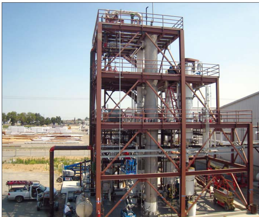
The distillation tower is located in the plant’s main yard.
